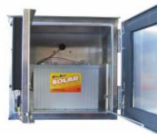
Battery is easily accessible.
